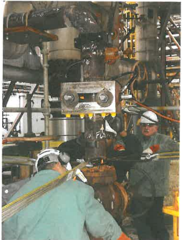
A crew at work on the steam system at the Plant 2 letdown station
